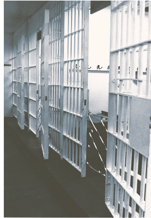
Image • Cells in the former Porter County Jail taken after it became home to the PoCo Muse.
