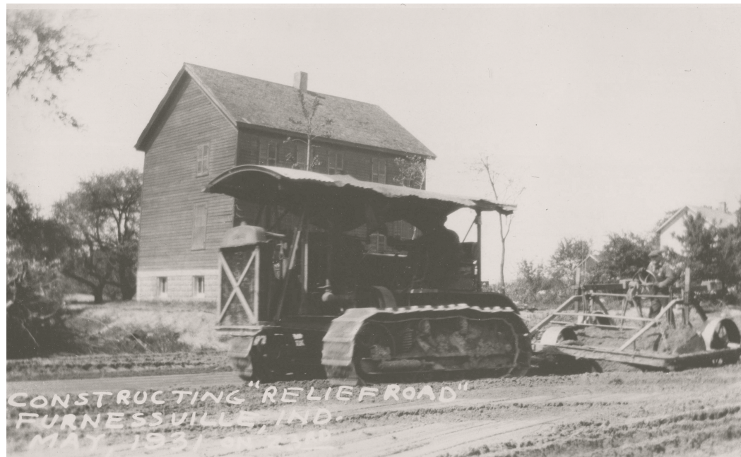
Above • An image of the “relief road” being constructed through Furnessville. May 1931. Right • The Williams’ Homestead before its relocation during the construction. May 4, 1930.
